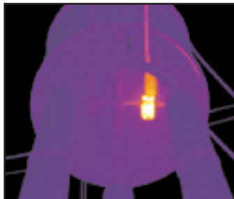
Overheat in power transformer
